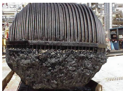
Typical fouled exchanger pulled prior to hydro-blasting operations
